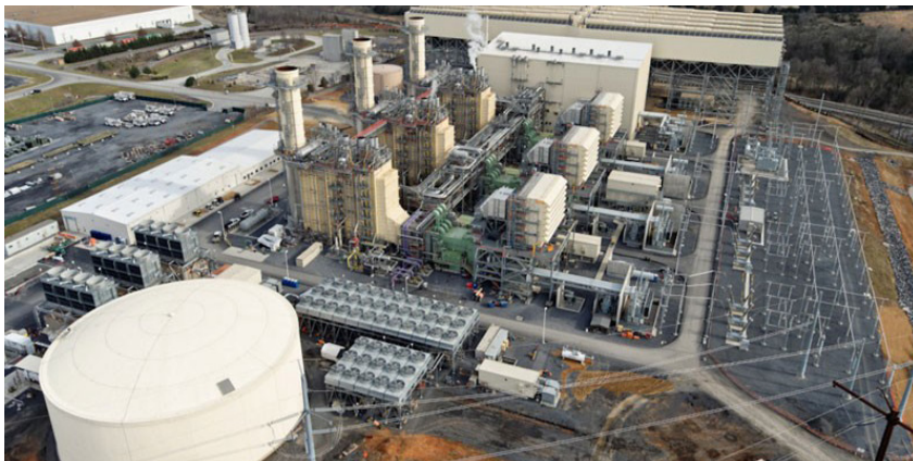
Warren County 3 x MHI 501GAC - 107 MW Added - 23,700 chiller tons - 8.9 MG tank
